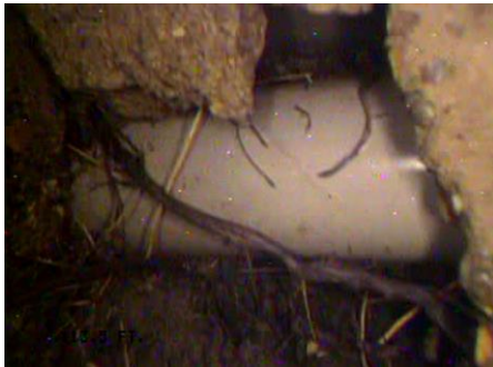
Section of Pipe Wall Missing, Exposed Line (113.5 ft.)
