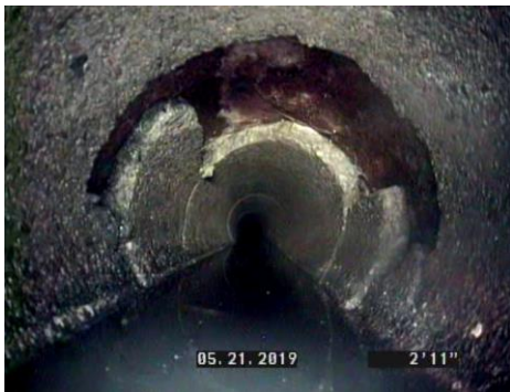
Broken Pipe with Visible Signs of Repair (2.9 ft.)
