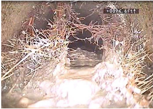
Major Root Blockage (94.6 ft.)
