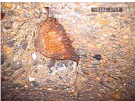
Fracture at Top of Pipe (284.4 ft.)
