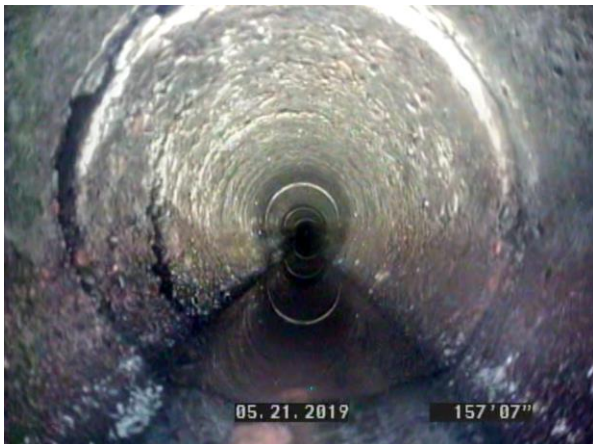
Circumferential Cracks in Pipe Wall (157 ft.)
