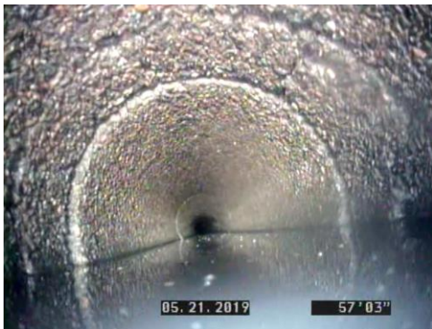
Circumferential Crack in Pipe (57 ft.)
