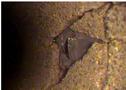
Missing Section in Top of Pipe Along with Fractures (88.7 ft.)
