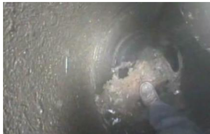
Steady leakage directly underneath dual 6-inch inverted siphon pipes.
