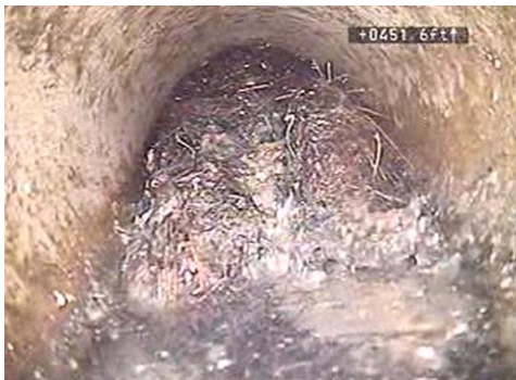
Complete Root and Solid Waste Blockage (451.6 ft.)
