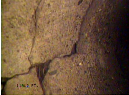
Fractured Pipe Wall (110.2 ft.)
