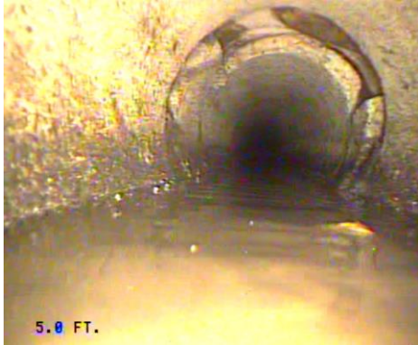
Broken Pipe with Repair Above (5.0 ft.)
