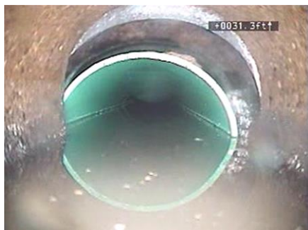
Disjointed PVC Pipe, Exposed Gasket (31.3 ft.)
