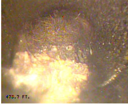
Major Root and Solid Waste Blockage (473.7 ft.)
