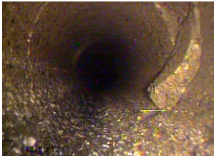
Protruding Concrete Wall (63.5 ft.)
