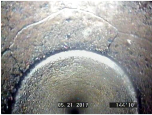
Cracking Near Joint (144.8 ft.)
