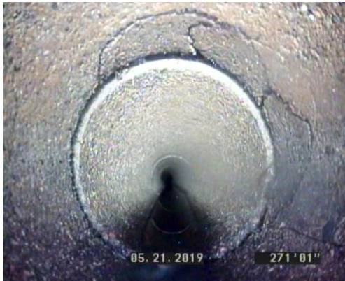
Cracking Near Joint (271 ft.)
