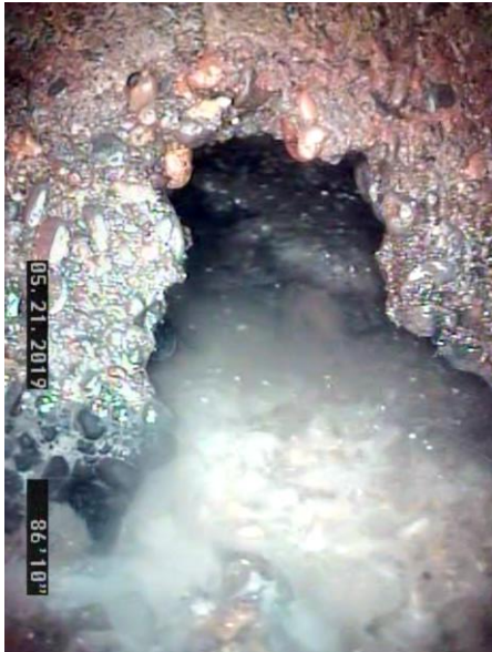
Large Crack in Pipe Exposing Outside Soil (86.8 ft.)
