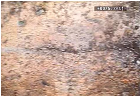
Fracture around Circumference of Pipe (75.7 ft.)
