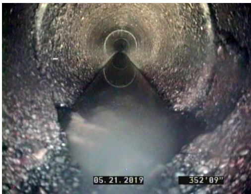
Broken Bottom of Pipe (352 ft.)
