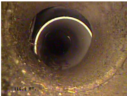
Disjointed PVC and Concrete Pipe Connection (116.1 ft.)
