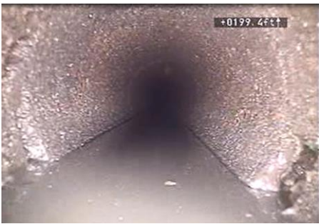
Holes in Pipe Joint on Either Side (199.4 ft.)
