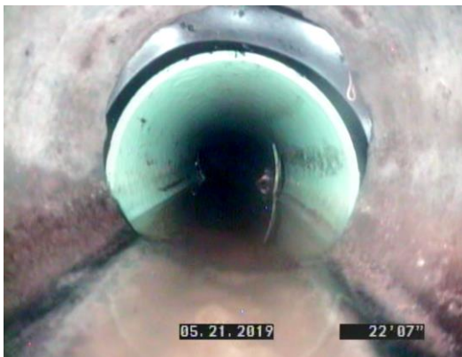
Disjointed Concrete / PVC Connection (22 ft.)
