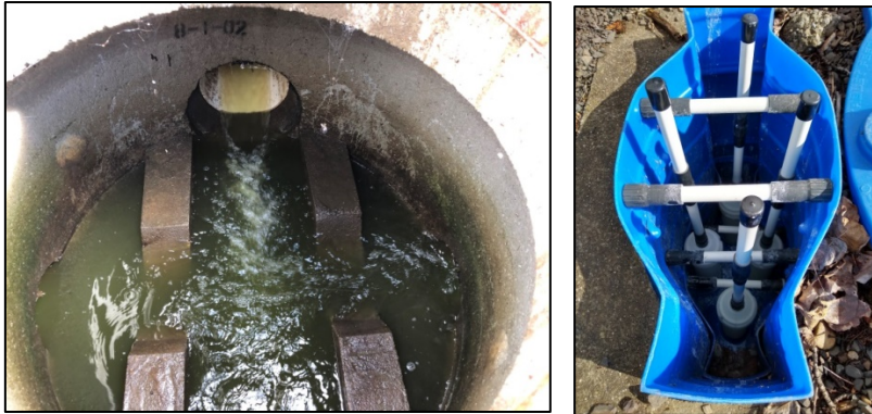
FIGURE 2.3.15 SODIUM HYPOCHLORITE STATION
