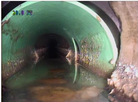
Disjointed PVC and Concrete Pipes (28.8 ft.)
