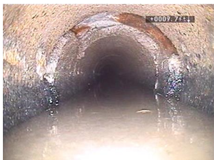
Broken Top of Concrete Pipe
