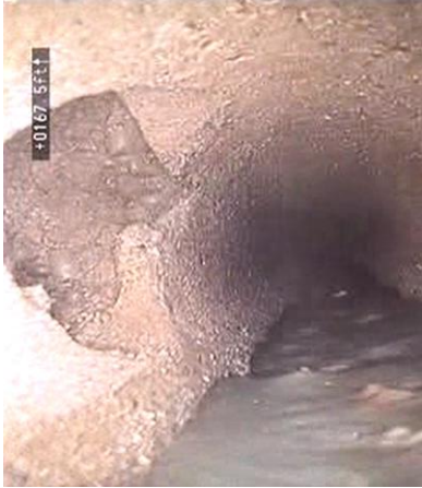
Broken Section of Pipe Wall (167.5 ft.)
