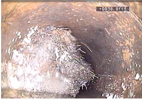
Major Root Blockage (38.8 ft.)
