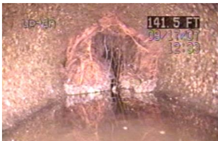
Significant Root Blockage (141.5 ft.)
