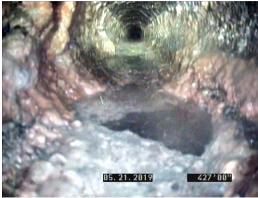
Buildup inside Pipe, Large Hole in Bottom of Pipe at Cleanout Location (427 ft.)
