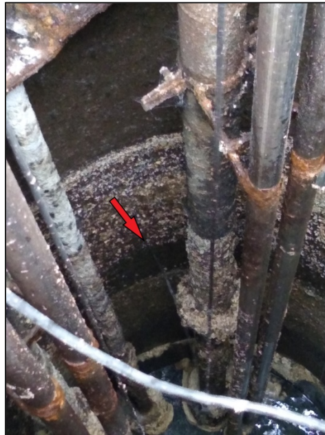
FIGURE 4.2.2 WATER INFILTRATION IN BEECH STREET PUMP STATION
