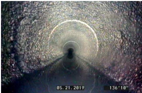
Cracks in Pipe Wall (136.8 ft.)
