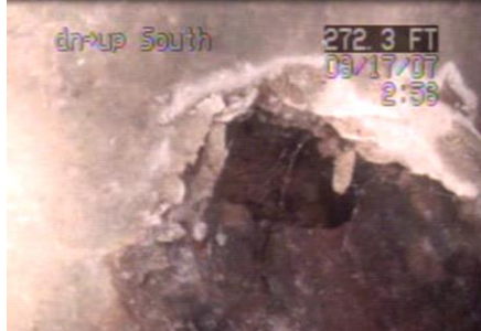
Broken Pipe Wall (272.3 ft.)
