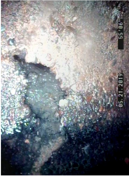
Crack in Pipe Exposing Soil (55 ft.)
