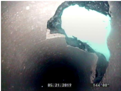
Broken Pipe at Cleanout Location (144 ft.)
