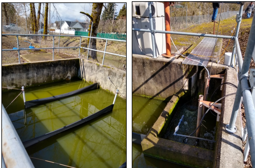
FIGURE 2.3.14 CHLORINE CONTACT BASIN
