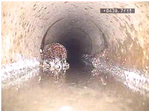
Root Masses Protruding into Pipe (438.7 ft.)
