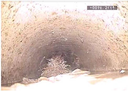
Heavy Root Blockage (96.2 ft.)
